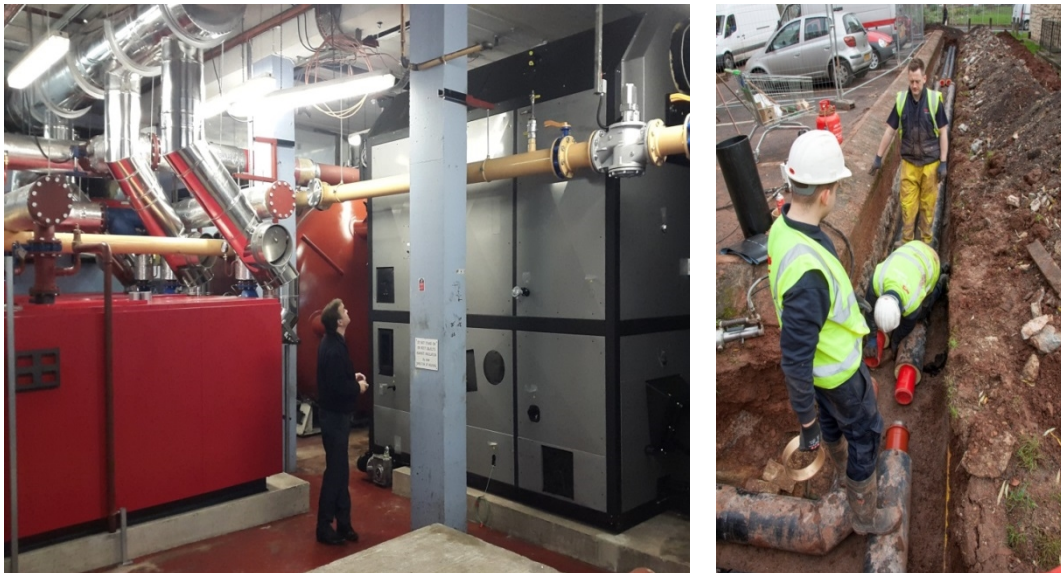
Figure 1 – Broughton House Energy Centre and installation of heat network between Broughton and Canynge.
